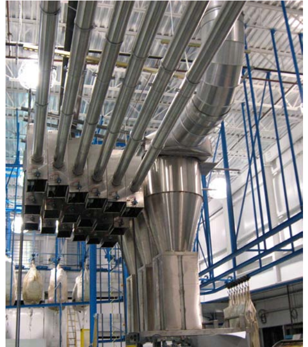
Accumulator bins with roof-mounted vacuum motor
