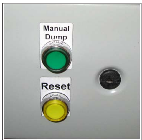
Individual Bin Controls
